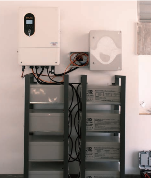
X3-NEO-LV & LEAD ACID BATTERY
